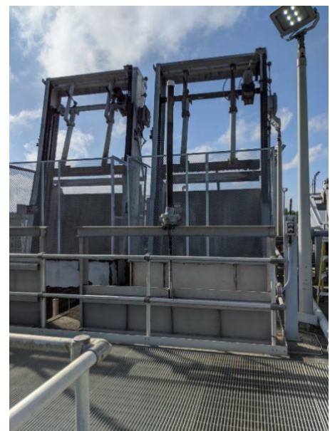
Bar Screens 3 and 4 in Need of Replacement
