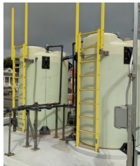
Bulk Fluoride Storage Tanks
