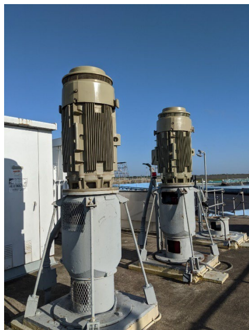
New High-Efficiency Motor on RAS Pumps
