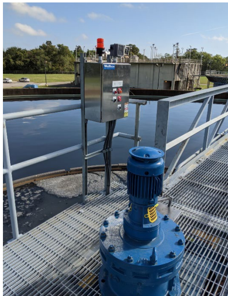
New Drive Unit on Primary Clarifier 1
